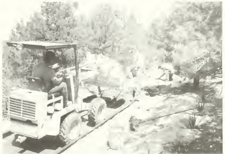
BLM engineers oversee design, construction, and maintenance of buildings, roads, and other facilities. Here a concrete trail is built to provide access to ANASAZI ruins.
